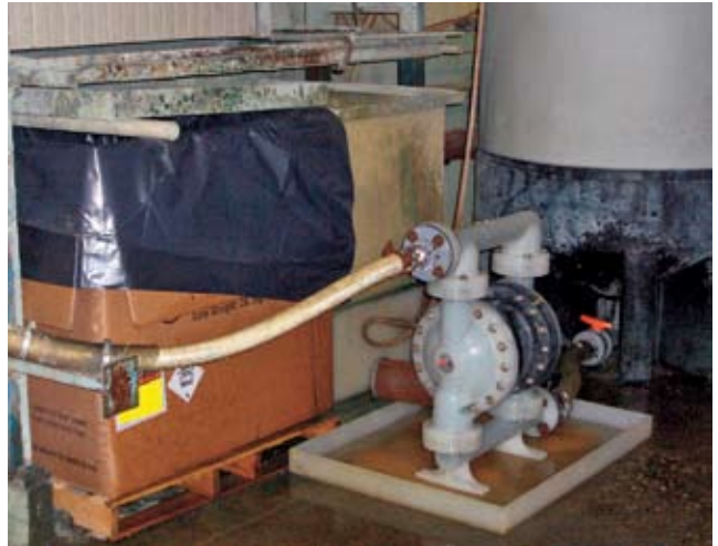
The rinse waters at CMF contain nickel, zinc and other acidic metals. After these rinse waters are treated and their chemistries adjusted to a neutral pH level, evaporators boil off the remaining water.
